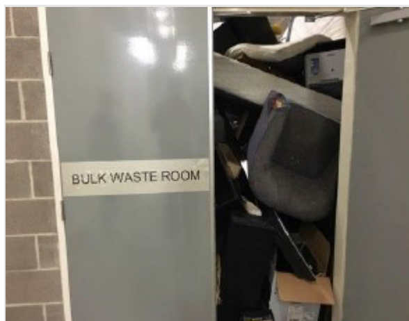
Image 3: inadequately sized bulky waste storage room.
